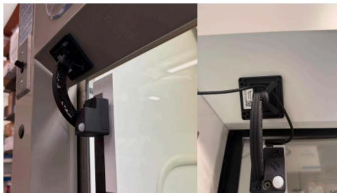
Figure 1. Installed Sashimi Sensors that Monitor Fume Hood Sash Height. Examples of the physical placement of the sensor unit on the fume hood exterior and the corresponding gradient strip.
