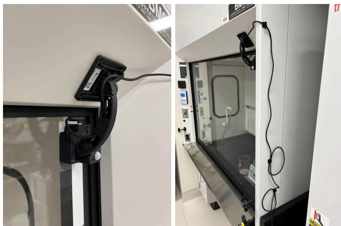
Figure 1. Installed Sashimi Sensors that Monitor Fume Hood Sash Height. Examples of the physical placement of the sensor unit on the fume hood exterior and the corresponding gradient strip.
